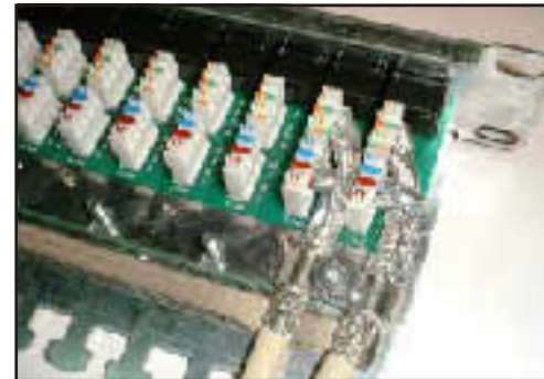
6. After termination completed. Please make sure the aluminum foil fully covers the wires.
