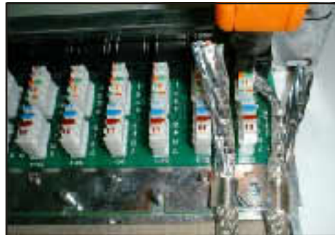
5. Arrange the wires according to the color and use punch down tool terminate each pairs.)
